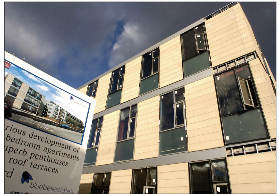
This £8.5m mixed development at Hopetoun Street in Edinburgh is the company's biggest contract to date.
